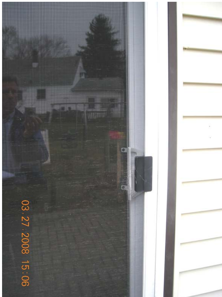
EXHIBIT 5 (Sliding Door – Broken Seal)
