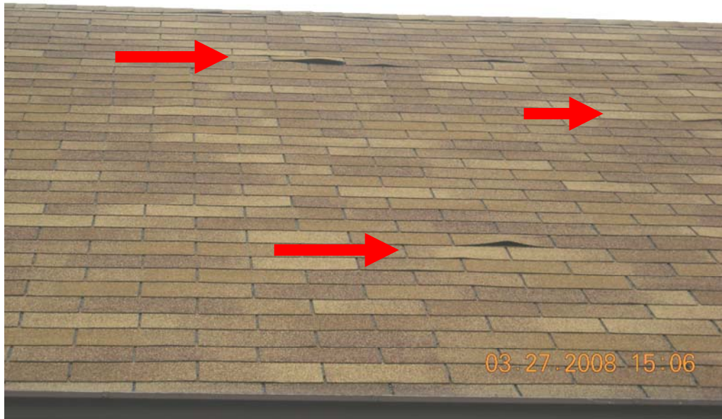
EXHIBIT 2 (Roof – Shingle Popping/Lifting Shingles)
