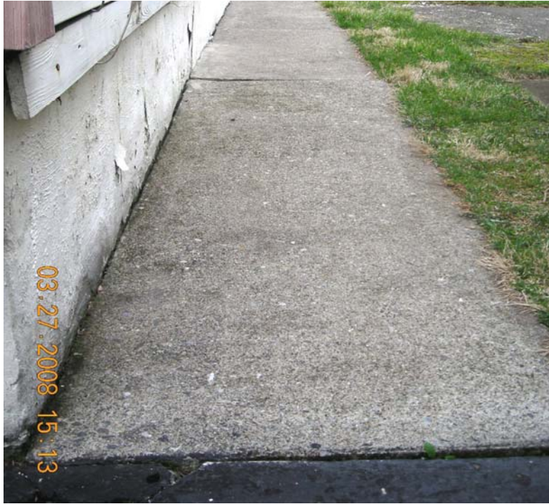
EXHIBIT 6 (Sidewalk – Slope Toward House)
