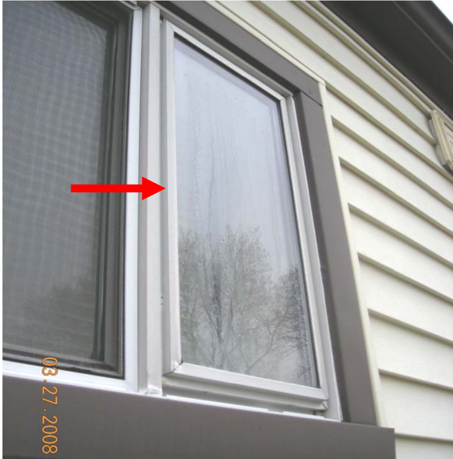
EXHIBIT 3 (Window – Broken Seal)
