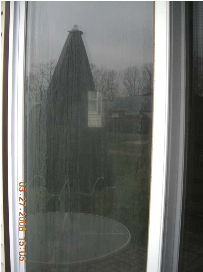
EXHIBIT 4 (Sliding Door – Broken Seal)
