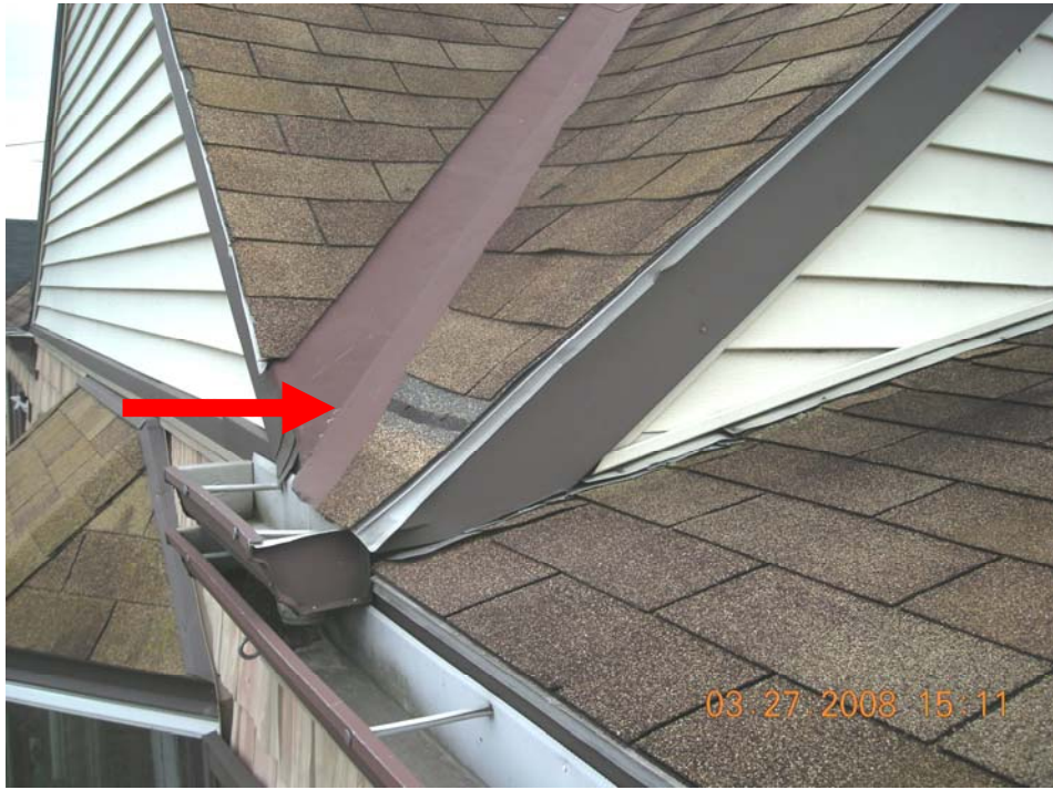
EXHIBIT 1 (Roof – Missing Shingle)
